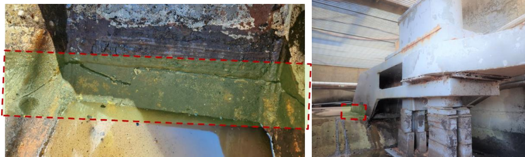
Figure 5: Location of crack at Boggs Lock and Dam
