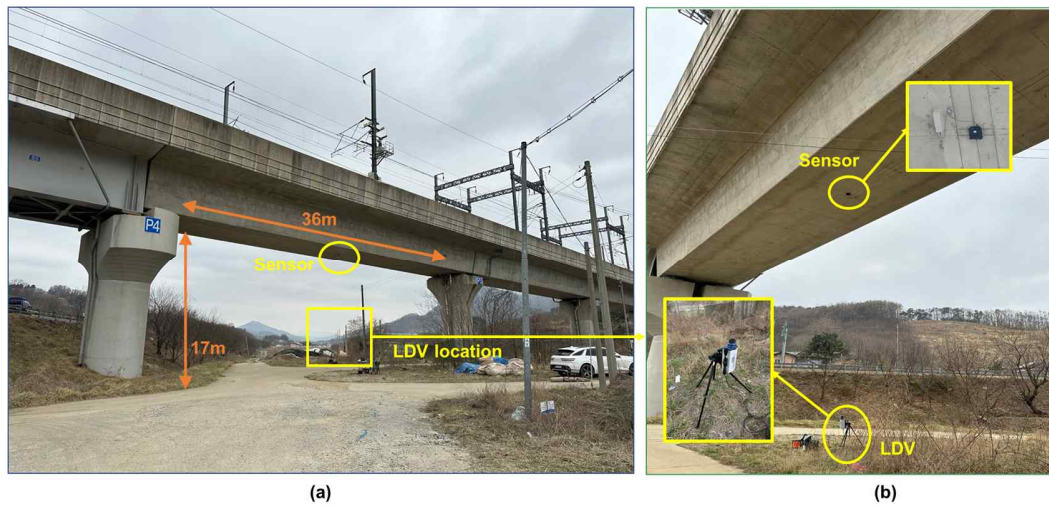
Figure 3. Experimental setup on the Gongju-Osong High-Speed Rail Bridge: (a) Elevation view indicating sensor positions and the Laser Doppler Vibrometer (LDV) reference measurement location, along with relevant distances. (b) Detailed illustration showing precise sensor installation and alignment beneath the bridge structure.
