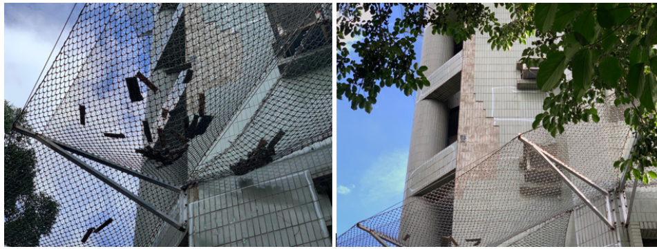
Figure 1. Challenges in current facade inspection methods.
