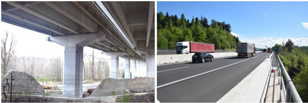
Figure 1. Case study viaduct: View from below (left) and view from above (right).
